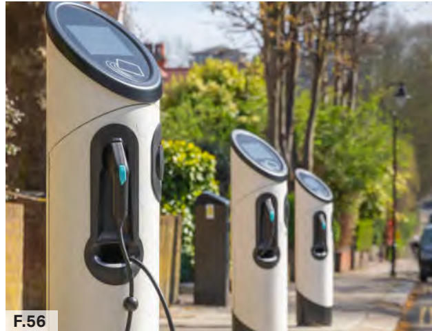
Figure 56: Examples of on-street car charging points.
