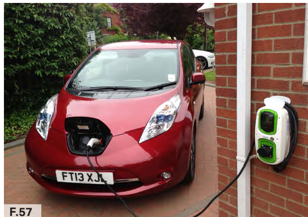
Figure 57: Examples of off-street mounted car charging points.
